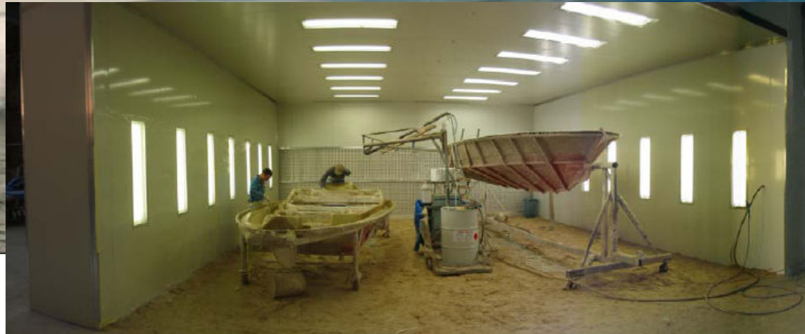
Oversized Industrial Painting / Fiberglass Booth – Solvent and Resin Fume Extraction
